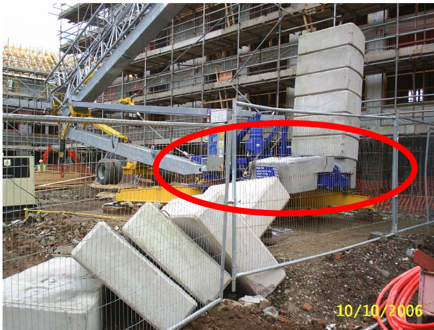
Photo 1 Crack in concrete and fallen ballast blocks.
