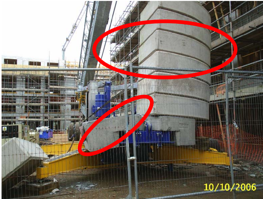
Photo 2 Crack in concrete and unstable ballast blocks.
